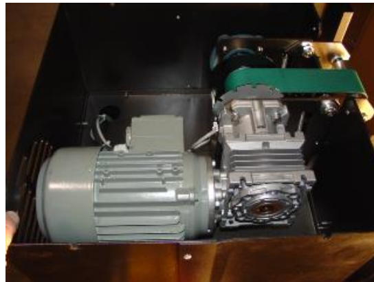
Check motor-replace if required
